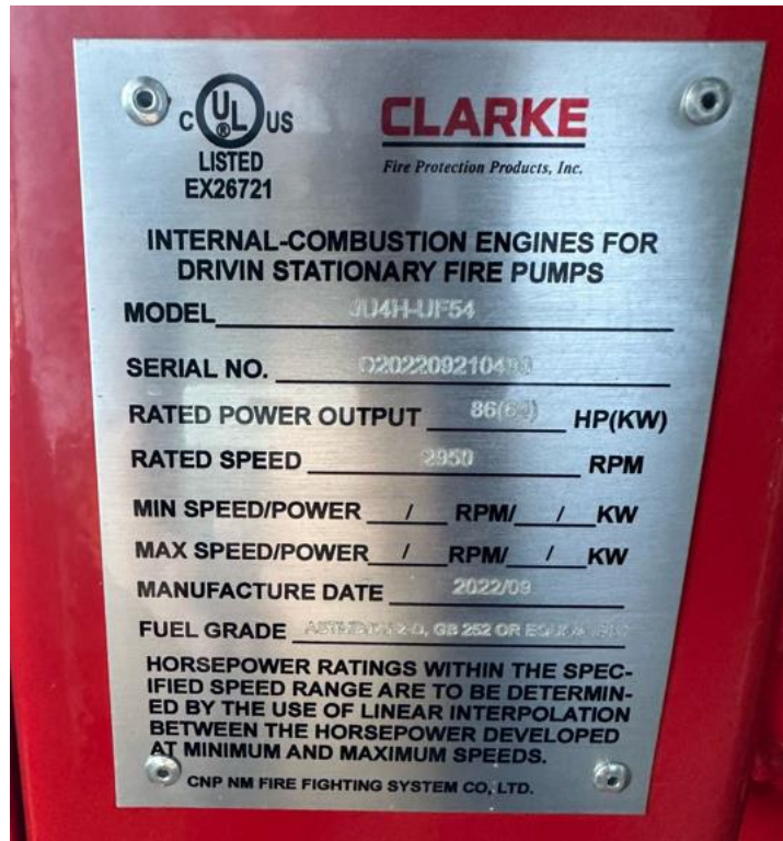
Figure 1. Photograph of the suspected counterfeit nameplate. A valid Clarke Fire Protection Products' nameplate would have the FM Approvals certification mark and a QR code present. It would not have a reference to CNP NM Fire Fighting System Co., Ltd at the bottom.
